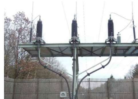
OHL cable terminations
