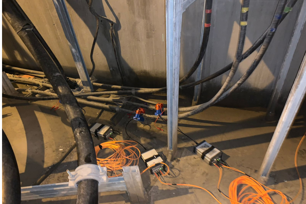
TR cable side HV/LV
